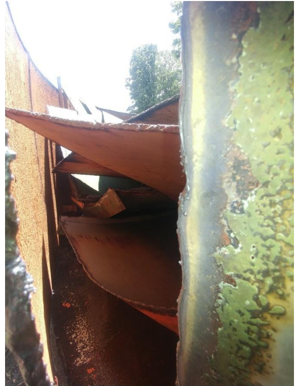
Panels Inside Tank.
