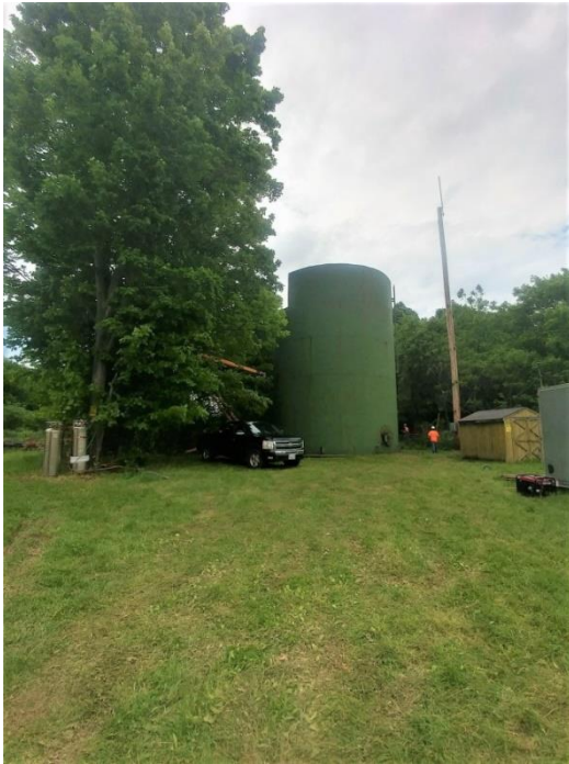
Roof Dropped Inside Tank.
