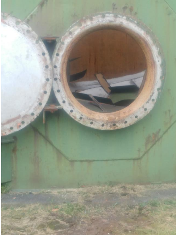
Panels Inside Tank.
